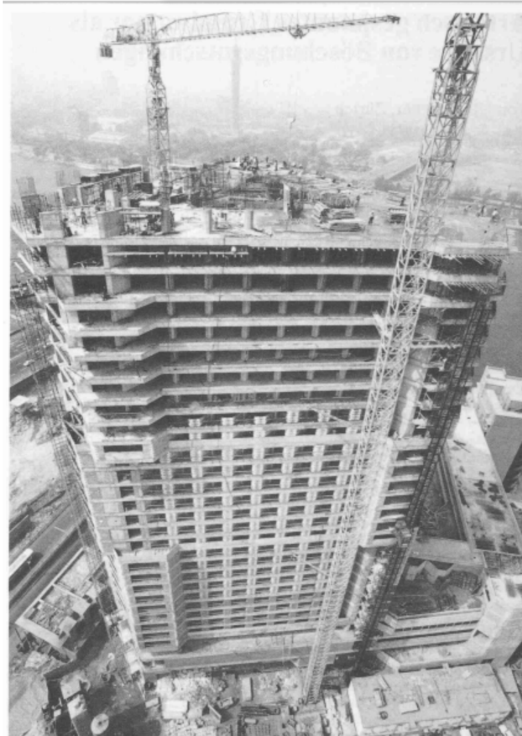
Fig. 1: Concrete work on the 26 th floor. In the background are the Nile and Cairo Tower. 25
